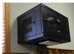
Internet internal connections upgrades
